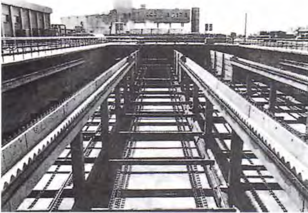
Sewage Treatment Plant
